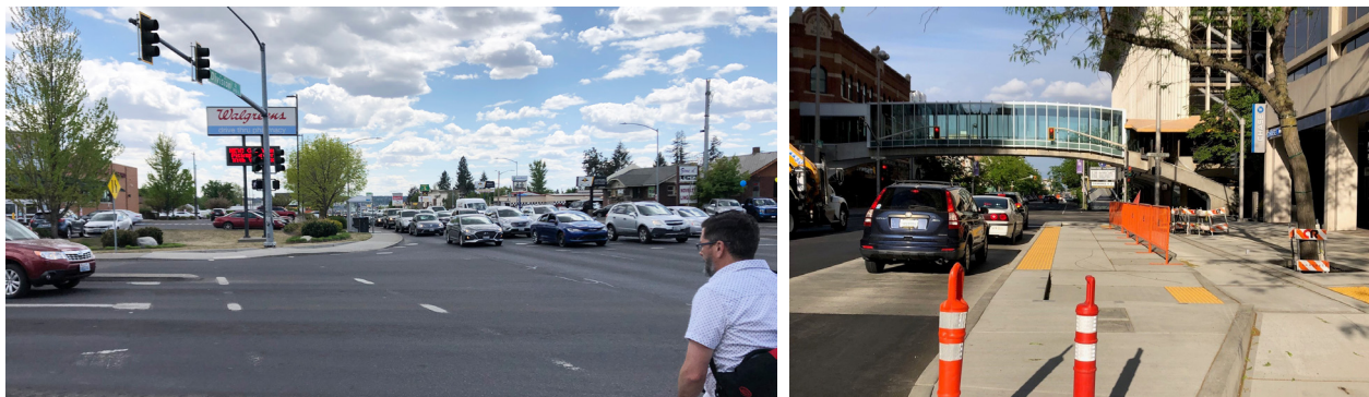
Left: Wide auto-oriented corridor as seen from Empire Avenue; Right: Construction of a new City Line island station and bicycle lanes in Downtown Spokane near Howard Street. (Credit: Parametrix)
